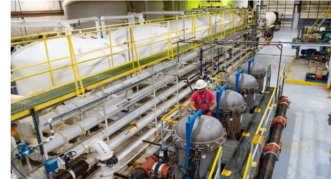
Christensen Satellite Plant Interior
