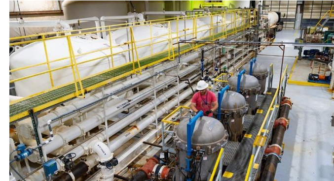
Christensen Satellite Plant Interior
