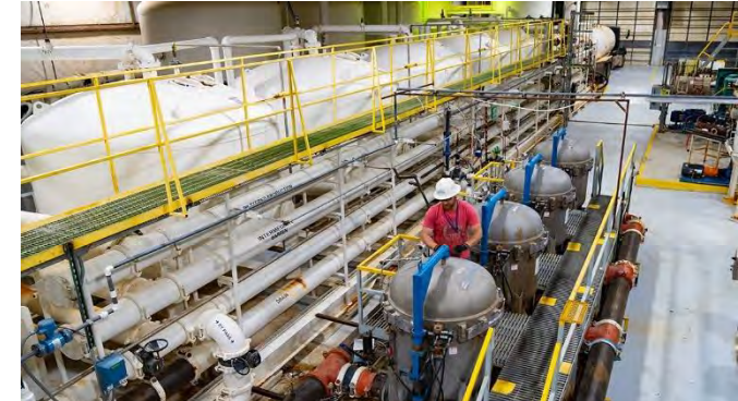
Christensen Satellite Plant Interior
